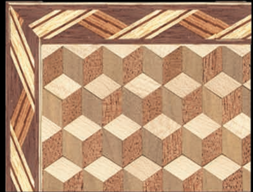
The decorative border has not been correctly applied and does not line up
