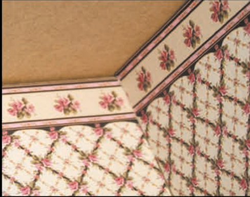
The wallpaper doesn't reach the ceiling. The design doesn't line up correctly
